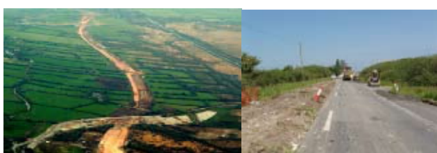
(1)The old A30 bisecting the Goss Moor SAC & new A30 being constructed (2) Downgrading the old A30 from a major trunk road to an access track.
