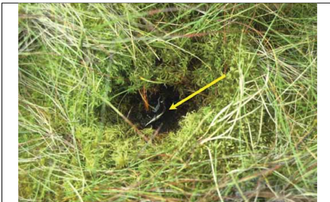
Figure 36. Overwhelmed sheet-steel dam in drain at Blawhorn Moss, Midlothian.
