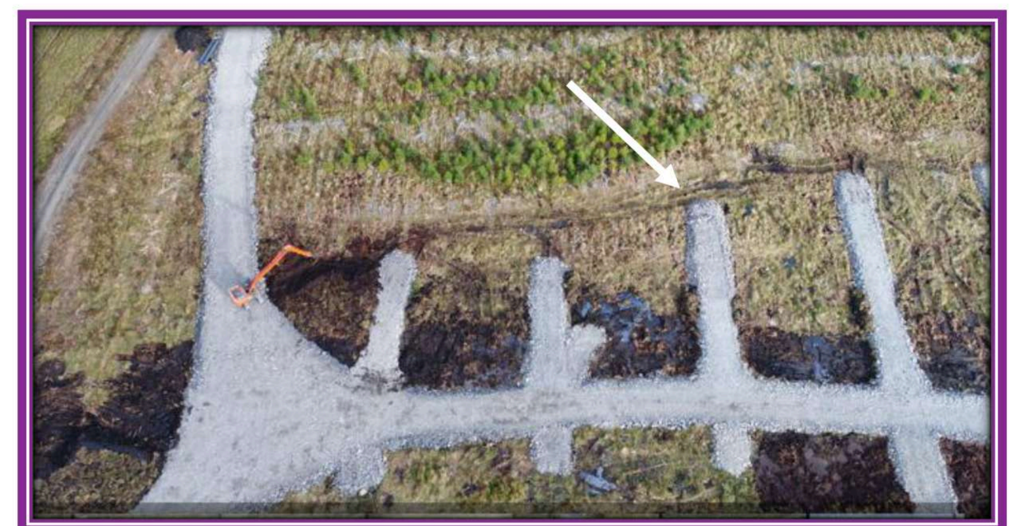
Picture 3: September 2025 – during reinstatement operation, spur roads were required to facilitate longer reinstatement reach, these were consequently buried with reinstated peat
