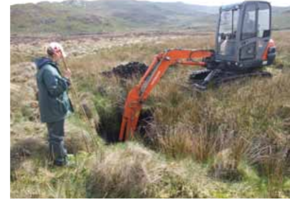
First suite of Pumlumon Project ditch blocking works being carried out on private farm land by a local contractor © MWT
