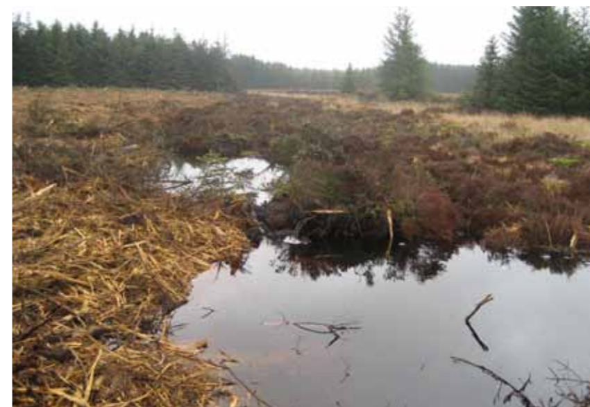
Following mulching of the tree tops, the forest drain has been blocked with a peat 'plug' © Forestry Commission
