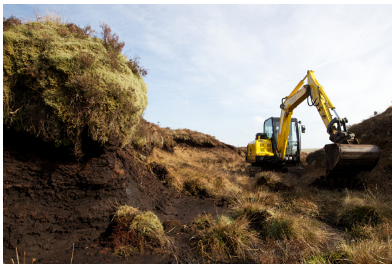
An excavator carrying out reprofiling work as part of restoration. Restoring our peatlands is vital for achieving net zero in the UK, but if it is done to mitigate for the carbon emissions associated with the development these savings cannot be included as a net gain in the national accounting. © Montgomeryshire Wildlife Trust
